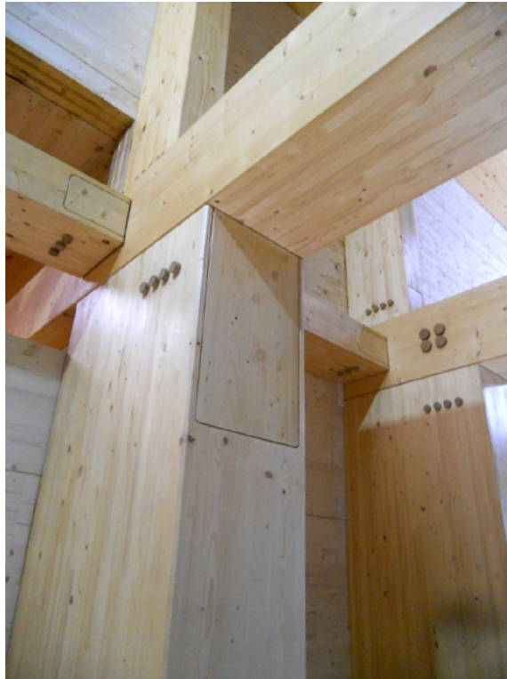
Fig. 2.28. Due to its better fire performance, timber conceals the steel beam-to-column connection – GlaxoSmithKline Carbon Neutral Laboratory for Sustainable Chemistry, University of Nottingham. © David Trujillo.
