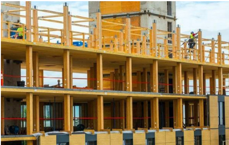
Fig. 1.10. Hybrid construction with glulam column and CLT beams. Source: Acron Ostry Architects. Photo: KK Law (cit. from InnoBYG, 2017).
