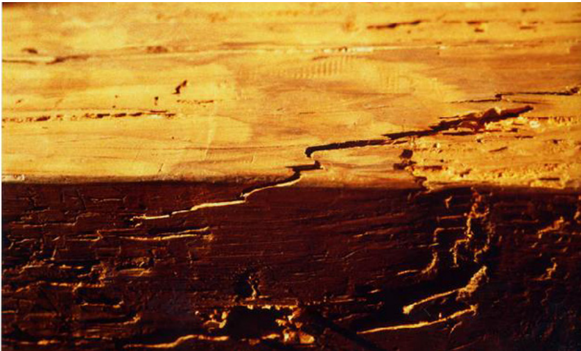
Fig. 6.37. Beam cracked by bending. The crack extends from the sides to the bottom edge (Tampone, 2007).
