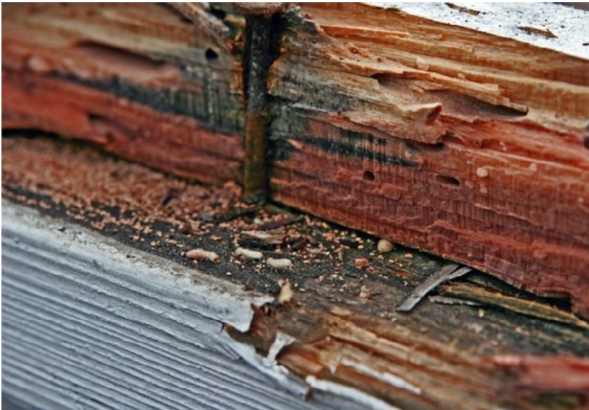
Fig. 6.32. Destruction of wood by termites (DC Scientific Pest Control, n.d.).
