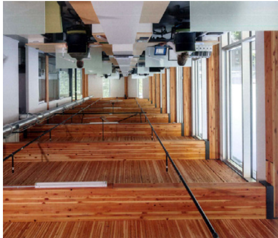
Fig. 3.40. Ventilation ducts under the load-bearing beams.
