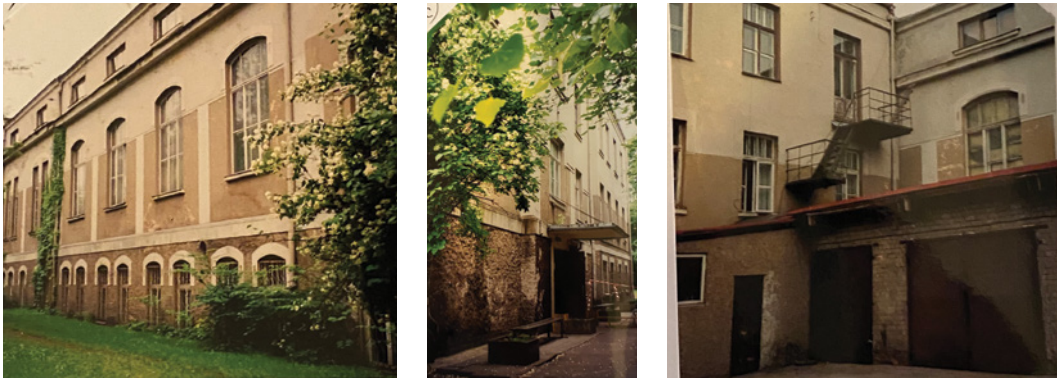
Figure 20. Photo fixations of the building at 7 Baldones Street before reconstruction: facade view from Vilpa Street ; facade view from Baldones Street ; facade view and the warehouse from the courtyard (2003).
