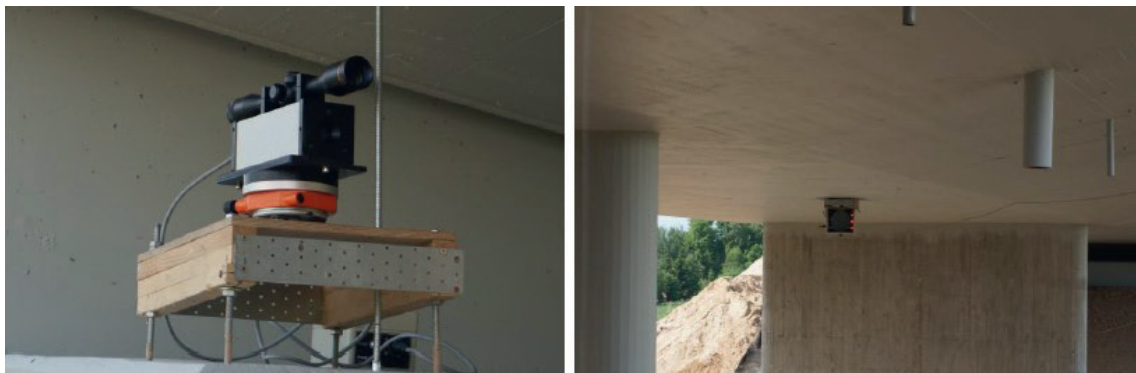
Fig. 1.2. The Noptel PSM-200 displacement sensor is installed on the bridge before performing a dynamic load test.
