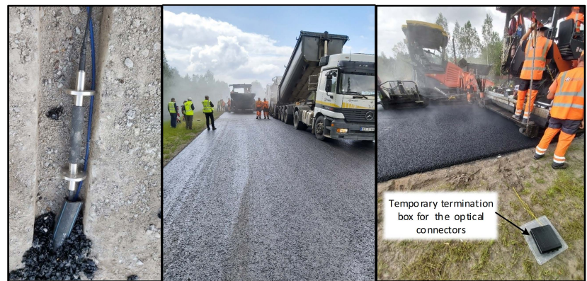
Figure 3. Photos from the construction process of road infrastructure where FBG sensors are integrated.
