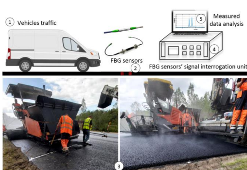
Fig. 1. Setup of FBG sensors integration and measurement process
