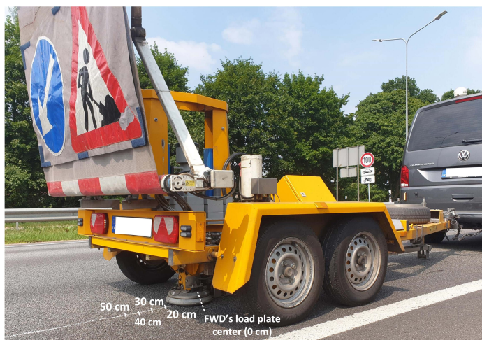
Figure 4. Realization of FWD experiments for calibration purposes of the embedded optical sensors.
